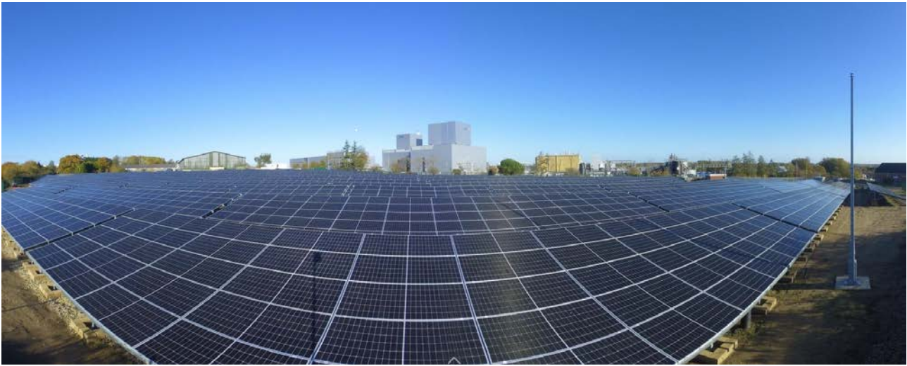
Haverhill solar farm operational in 2023
